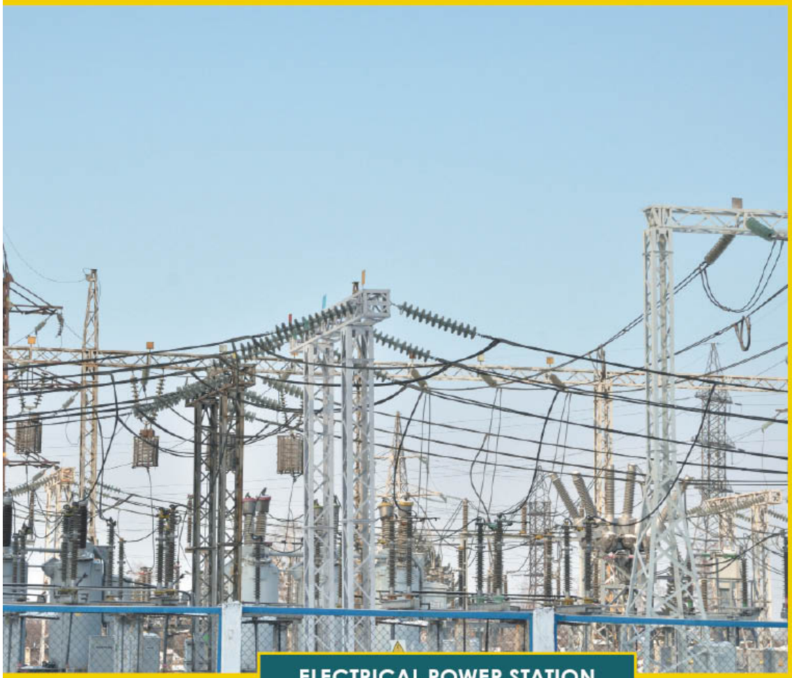
ELECTRICAL POWER STATION
