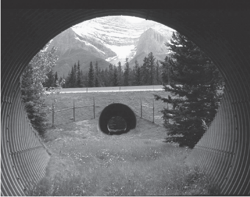
FIGURE 4.7 This culvert undercrossing is one of thirty-eight wildlife underpasses and six wildlife overpasses constructed because of concerns about the Trans-Canada Highway bisecting Banff National Park. (Photo by Anthony Clevenger.)
