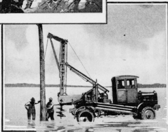
Everything from the bottom of the hole to the top of the pole, including a machine to dig the hole—Western Electric backs up the public utilities with all manner of supplies.
