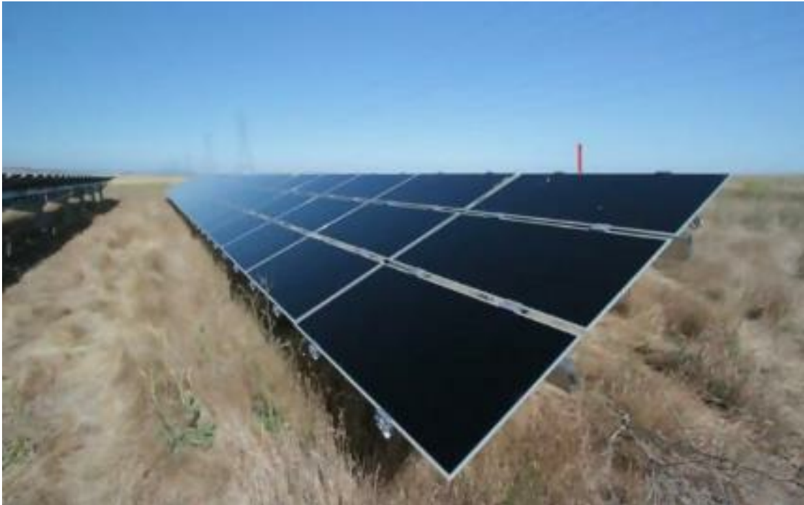
First solar PV modules installed in a 40-MW power plant Source: Renewables Now
