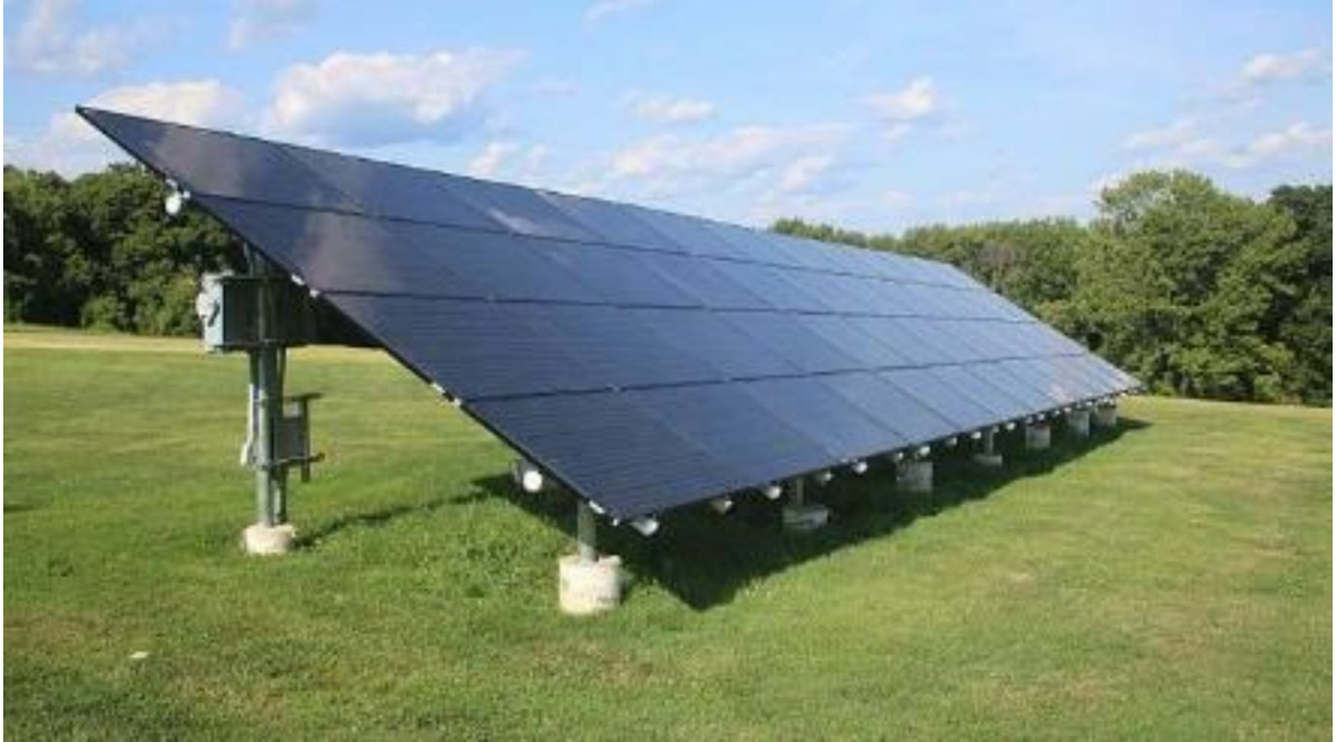
Ground-mounted solar panels Source: Wikimedia.org
