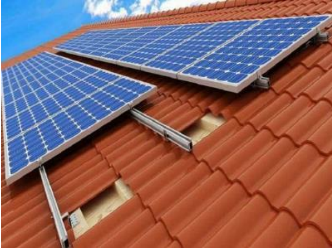
Solar panels mounted on rails Source: FOEN solar bracket
