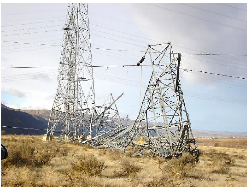
Figure J-1. Failure of a 230 kV lattice structure.
