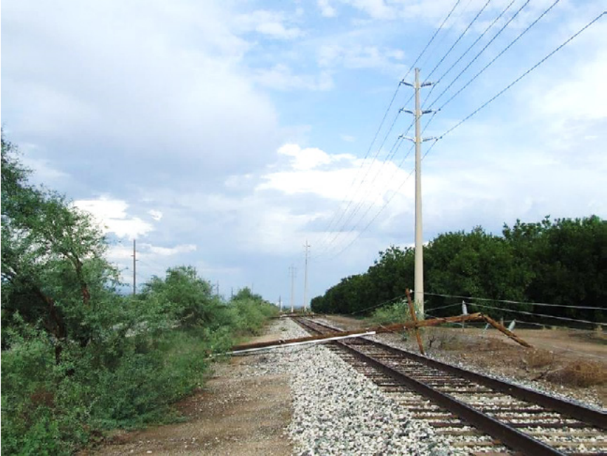
Figure J-3. Failure of a 46 kV wood pole line.
