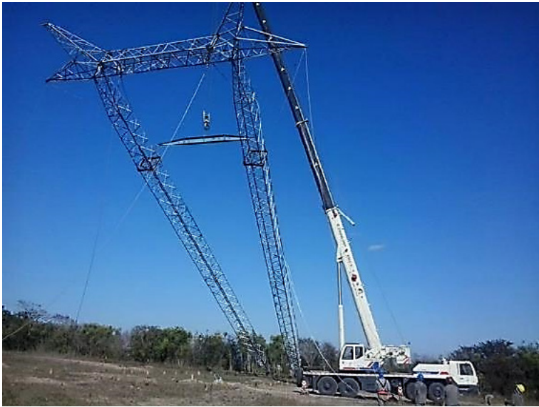
Figure 3-1. Structure erection of (a) a tubular steel H-frame structure; and (b) a latticed steel guyed tower.
