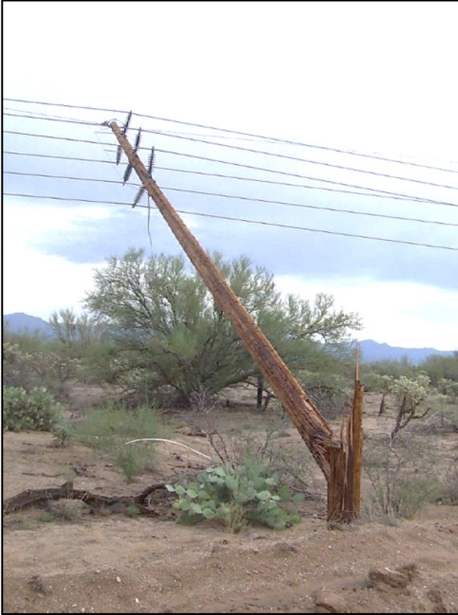
Figure J-2. Failure of a 46kV wood pole.
