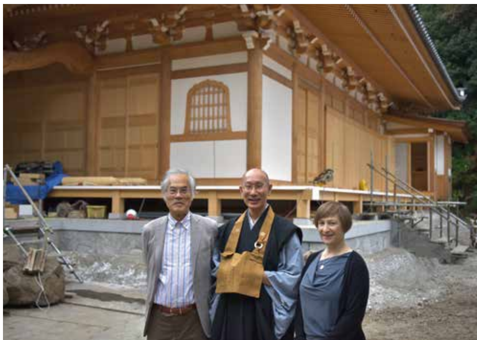
LEFT Terunobu Fujimori, Shunmyo Masuno, and Mira Locher visit the construction site of the almost completed new main hall for the Kenkohji temple in Yokohama, where Masuno serves as head priest.
