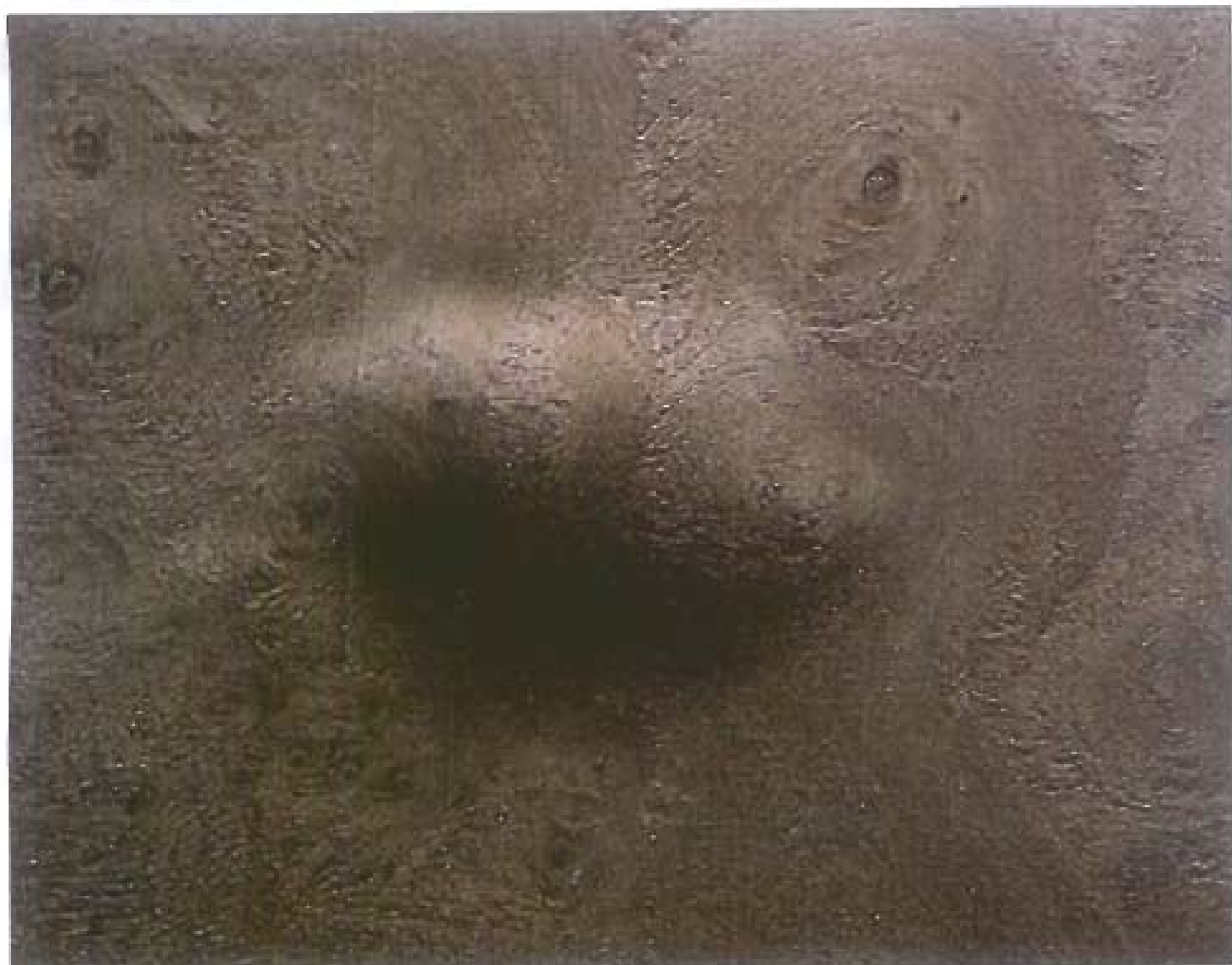
Blister caused by patchy application of glue.
