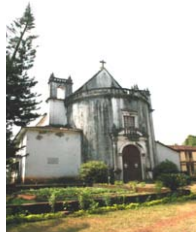
Fig. 5.130. Old Goa. Royal Chapel of Saint Anthony. 17 th Century. Laterite and mortar.
