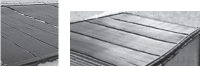
Figure 17: Installed unglazed collectors.
