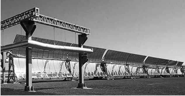
Figure 101: The molten-salt-cooled parabolic trough collector at ENEA, Casaccia, Rome.
