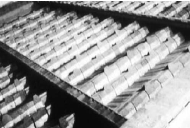
Figure 18: Switched off oven moving grate.
