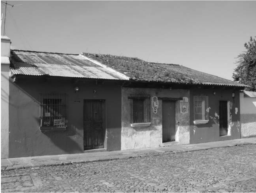
Illustration 1—Three Antigua houses in violation of UNESCO and city codes: one property split into three with corrugated steel and poorly maintained roofs. Photograph by the author
