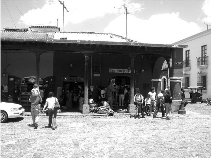
Illustration 2—The corner of the Portal on the Central Plaza in violation for having a corrugated-steel roof in poor repair. Note the kneeling vendors selling contrary to city officials' desires. Photograph by the author
