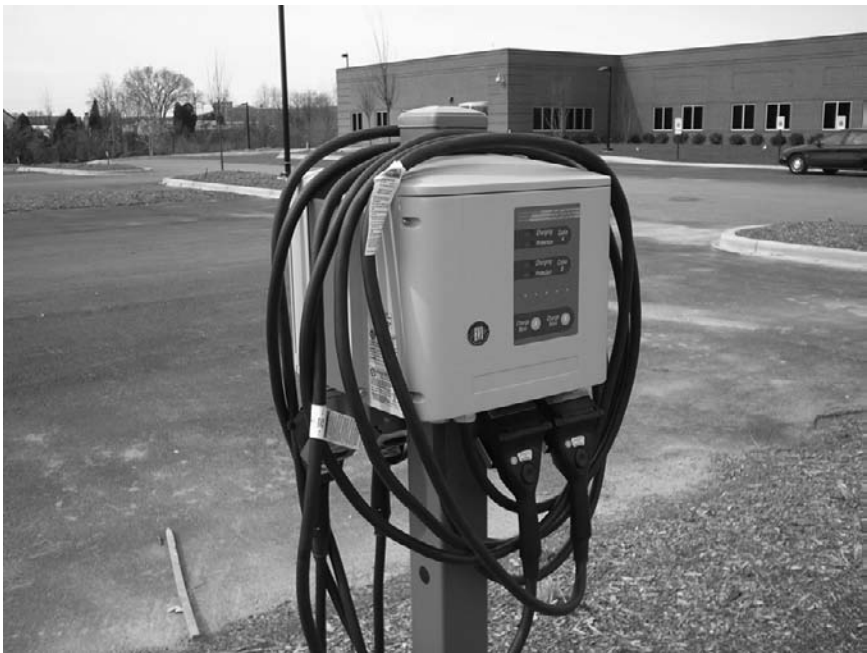
16-6. Recharging Station for Electric Vehicles
