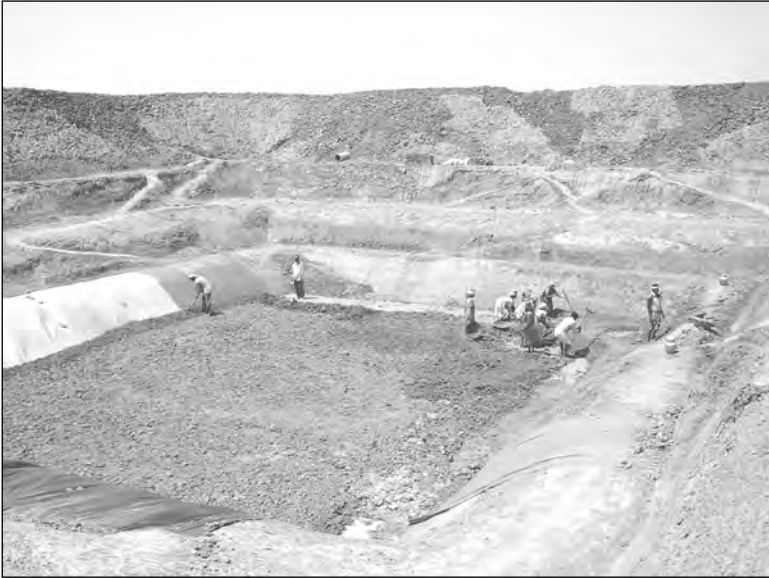
Plate 40.2 New tank at Kamia
