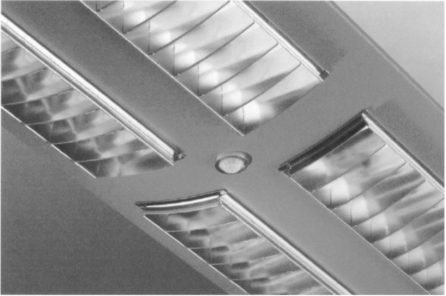
Figure 14-7. Suspended direct-indirect luminaires with integrated sensors can maximize energy savings in office applications. This integrated sensor provides both occupancy sensing as well as wireless personal dimming. The sensor can be configured to control only the downlight in cubicle spaces; in private offices, the sensor would control both the uplight and the downlight. The sensor is also compatible with DALI communications. Courtesy: Lightolier
