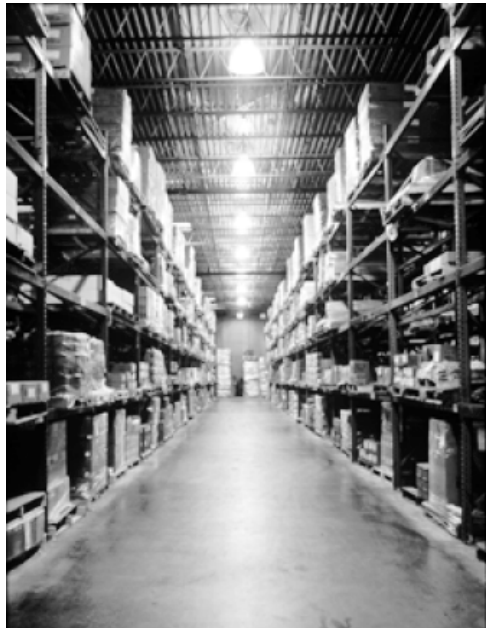
Figure 16-1. In warehouse aisles, lighting upgrades should maintain the target illuminance on vertical surfaces. This can be achieved with clear prismatic reflectors. Courtesy: Lithonia Lighting.
