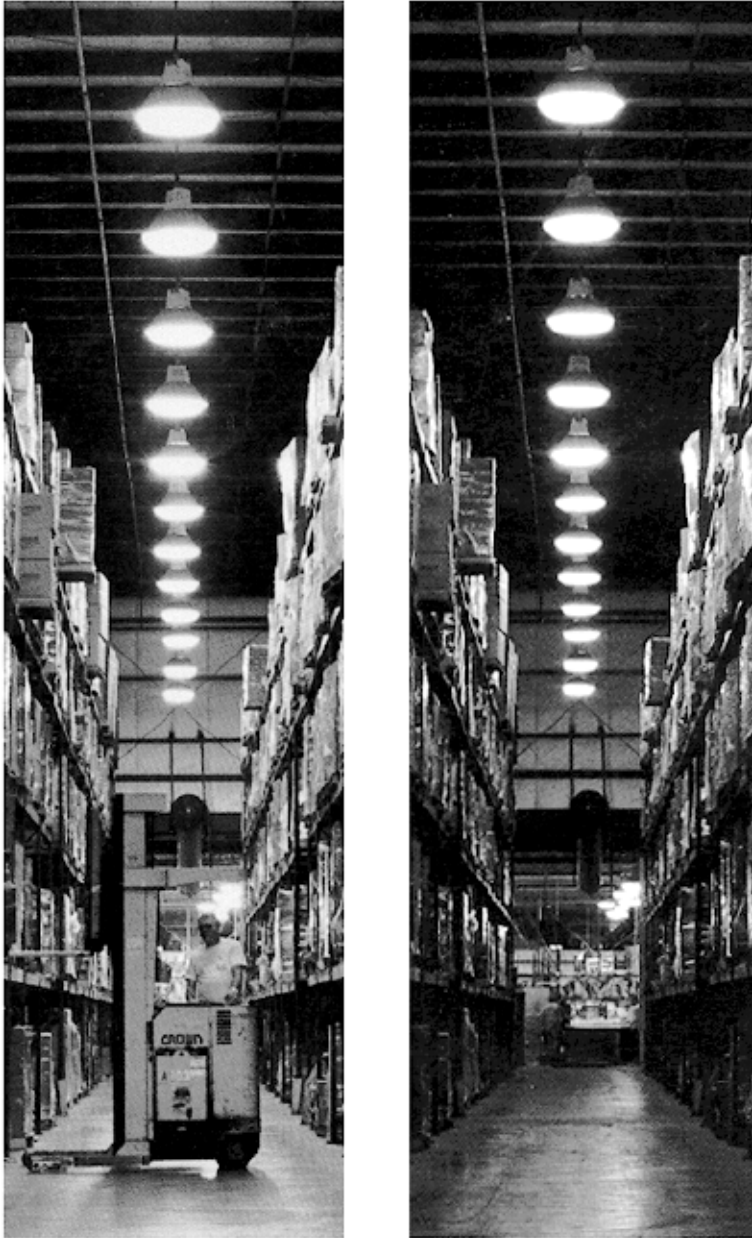
Figure 12-8. Bi-level HID switching systems can save energy by providing a low level of “standby” light output while the space is unoccupied. Courtesy: Thomas Lighting, Inc.
