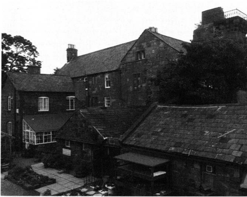
33 Brimstage Hall, Cheshire. A pattern of blocked windows and scarred walls reveals a complex story of building and rebuilding.
