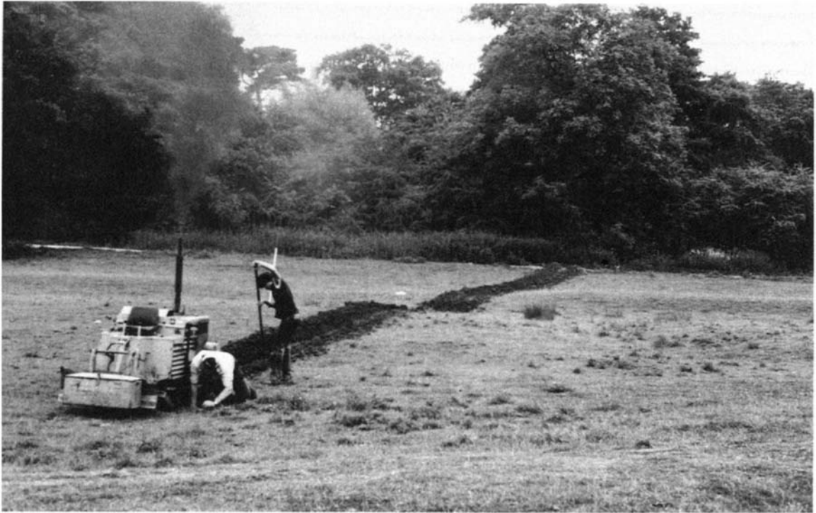
59 Keeping a careful eye on pipe-laying operations in the Abbey Meadows, Redditch.
