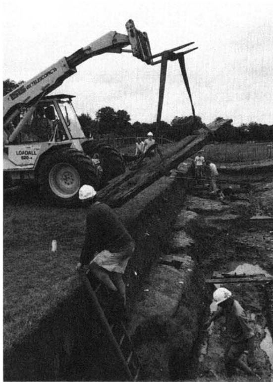
4 Bordesley Abbey industrial site, lifting the last timber from the earliest of the mill's tailraces.
