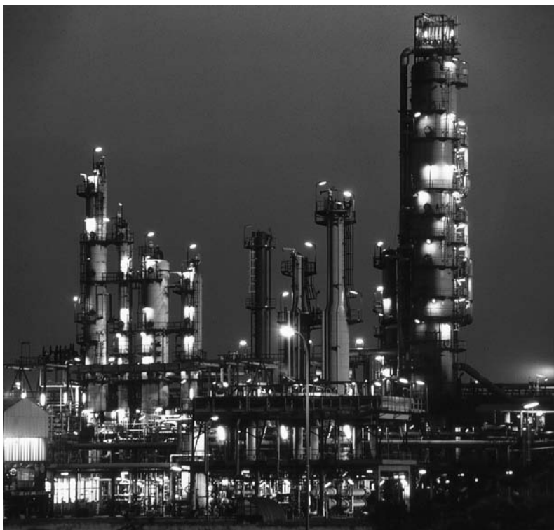
Figure 1. The distillation tower of an oil refinery
