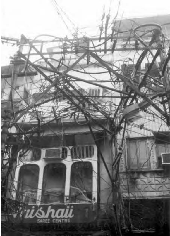
Figure 5.1 Grid failure in India
