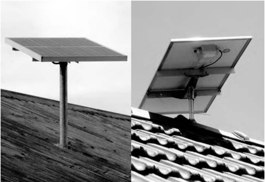
Figure 1.10 Installed solar PV modules (from above and below)
