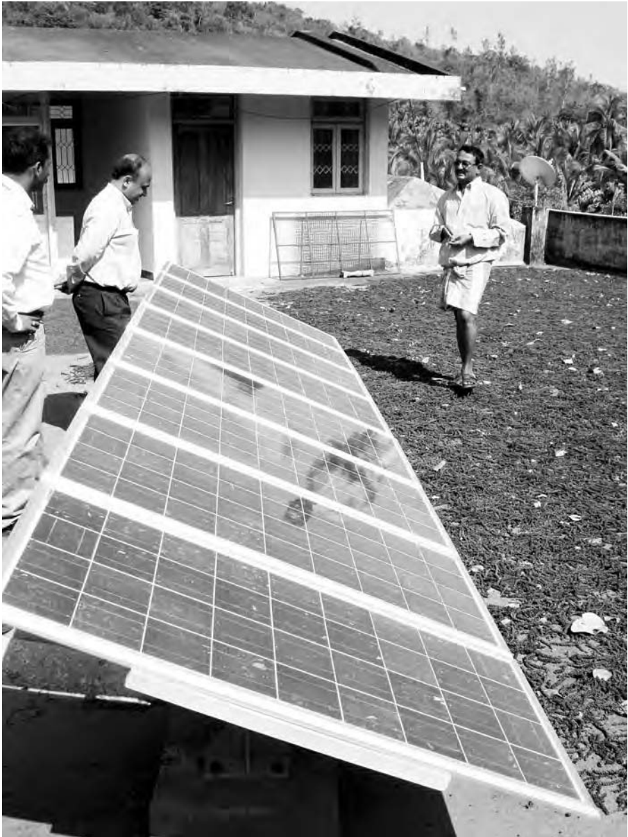
Figure 1.19 Larger solar system for appliances running on alternating current (AC)
