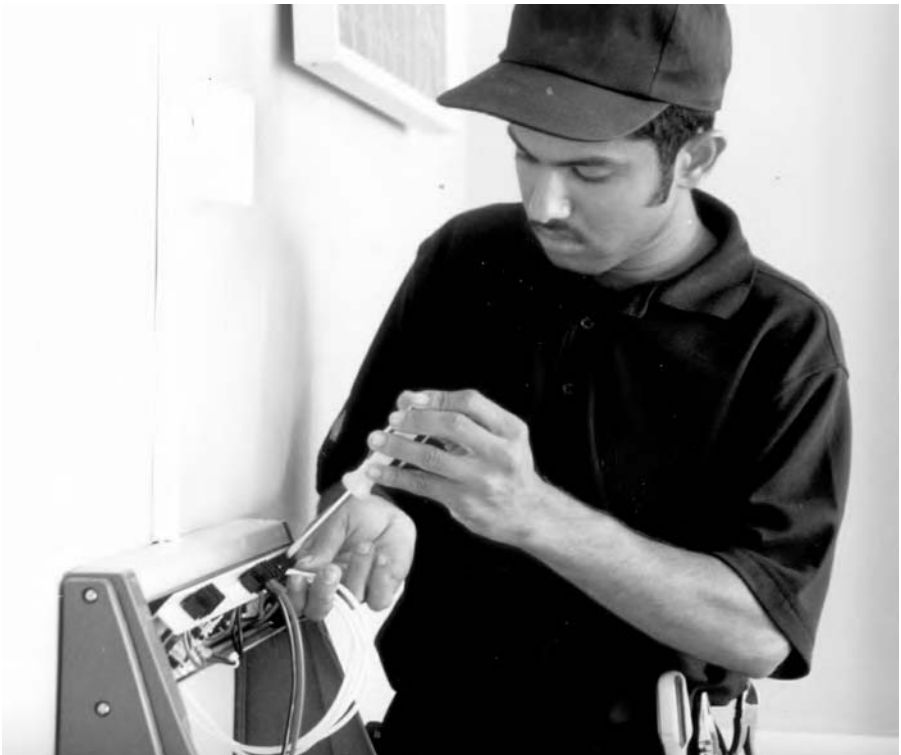
Figure 5.50 Wiring solar module to electronics and battery
