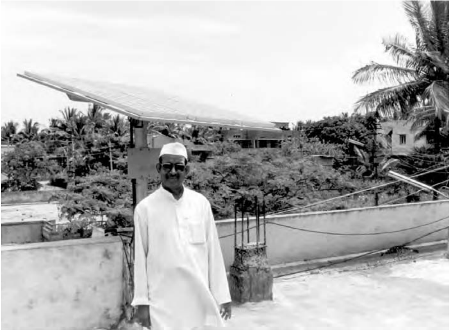
Figure 5.8 Larger solar installation in suburban setting
