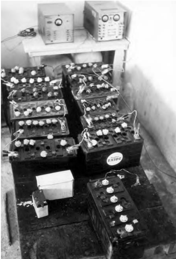
Figure 1.4 Typical battery-charging station in village
