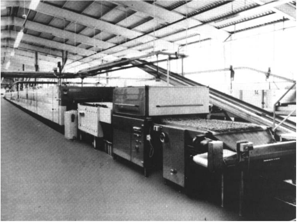
Fig. 16.5 Tunnel oven. (Courtesy of Werner and Pfeiderer Ltd.)
