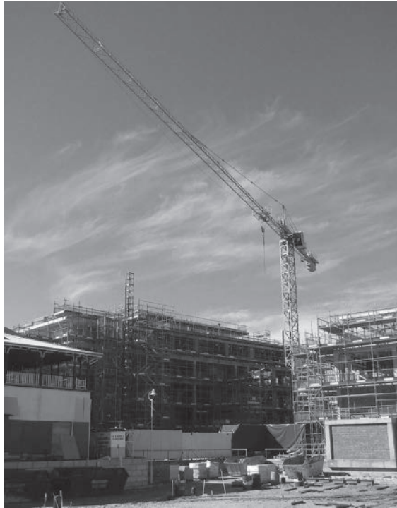
Figure 10.1 Unwritten tacit and implicit knowledge in engineering practice. Take a look at this construction site. How much of what you can see in the picture is shown in the drawings? Answer: not much, because the drawings show details of the finished building. They do not show all the steps needed to make it, such as in a LEGO instructions leaflet. For example, how did the builders know where to put the crane and how to construct the scaffolding? Those elements were not shown on the building drawings.
