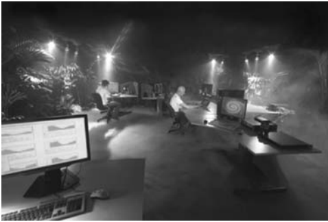
Figure 3.2. Bahnhof data center, Stockholm, Sweden.
