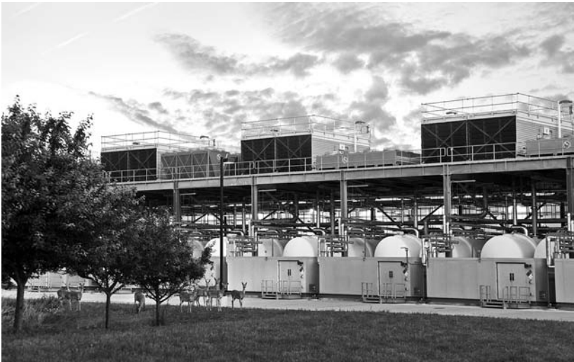
Figure 3.5. Council Bluffs, Iowa data center with deer in the foreground.
