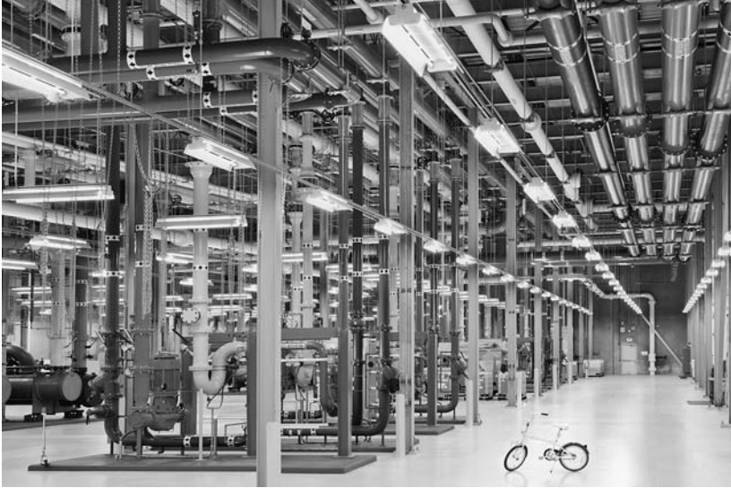
Figure 3.1. Douglas County, Georgia, data center. Shown here are colorful pipes distributing water for cooling the facility, and Google’s G-bike, the “vehicle of choice” for transportation in and around the data centers.
