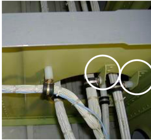
Figure 5.24. Support brackets highlighted in white circles, conducting harnesses through a machined frame. For a color version of this figure, see www.iste.co.uk/duvaut/IAM.zip
