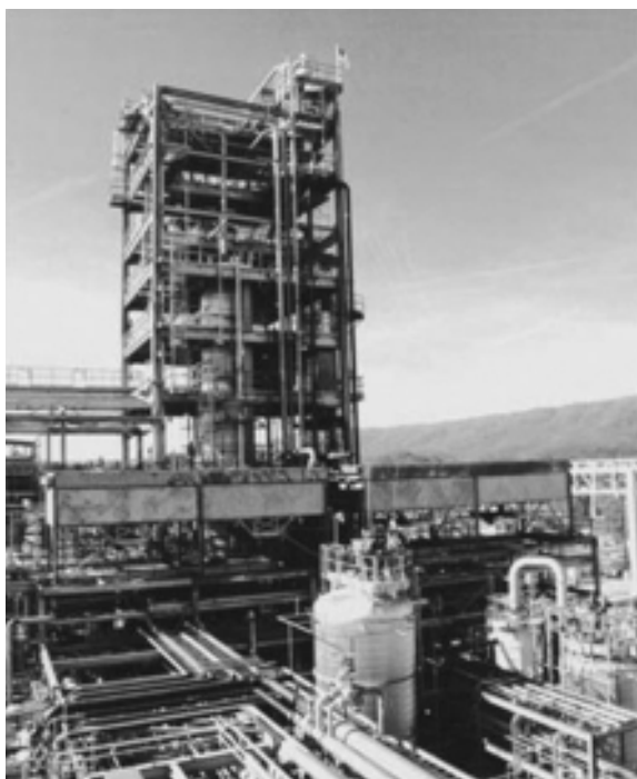
Figure 1.15. Air Products's LPMEOH process demonstration unit for methanol synthesis using syngas from coal gasification with slurry bubble column reactor, located at the Eastman Chemical site in Kingsport, Tennessee. U.S. DOE Topical Report No. 11, April 1999, under DOE contract #DE-FC22-92PC90543. Photo: courtesy of Debbie Bauer, Corporate Communications of Air Products.
