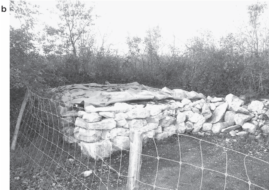
Fig. 6.1. Construction of an artificial site for winter retreat and egg-laying in Chizé Forest, France. (a) Construction process (b) Finished shelter site (with the upper sheeting pulled back to reveal construction details).
