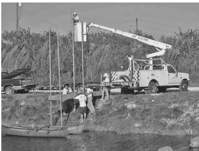
FIGURE 14.1 Building a surface water sampling dock and platform at a canal site.
