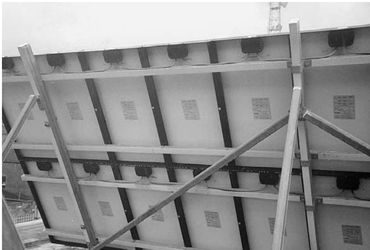
Figure 5.4 Junction boxes on a free-standing roof-mounted installation
