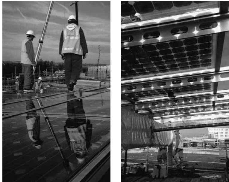
Figure 14.19 Details of the PV mounted on the atrium roof at the University of Nottingham
