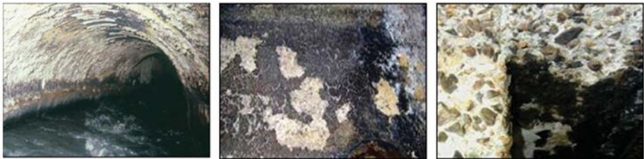
FIG. 14.2. – Image of a sewage pipe subject to different stages of biodeterioration.
