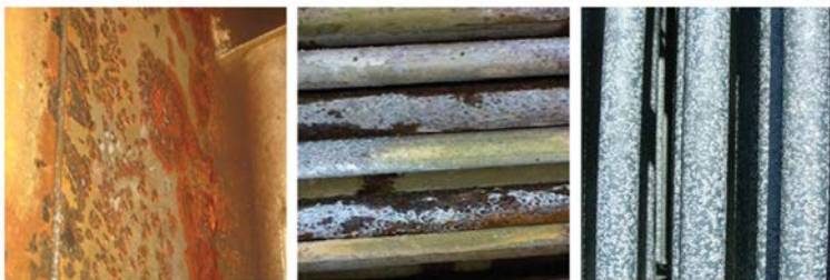
FIG. 9.9. – Corroded internal surfaces of cooling tower pool (on the left), a galvanized steel tubular exchanger (in the centre and on the right).
