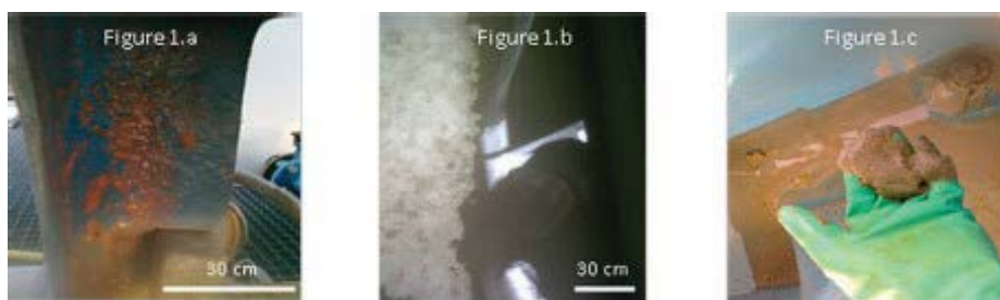
FIG. 9.2. – Diversity of the deposits observed in cooling circuits. 1.a: reddish deposit on the internal surface of the tower’s immersed plastic elements. 1.b: blackish deposit in the bottom of a cooling tower basin. 1.c: deposit recovered at the lowest point of a cooling tower basin after a chemical cleaning operation.
