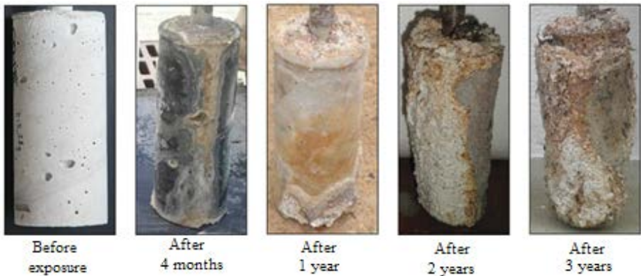
FIG. 14.11. – Typical evolution of the positive control for deterioration (CEM I + Silica sand) during 3 years of exposure on-site [38].
