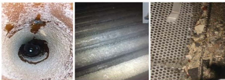
FIG. 9.8. – Scale deposits on the surfaces of pipework (on the left), tubular exchanger (in the centre) and at the bottom of the cooling tower's pool (on the right).
