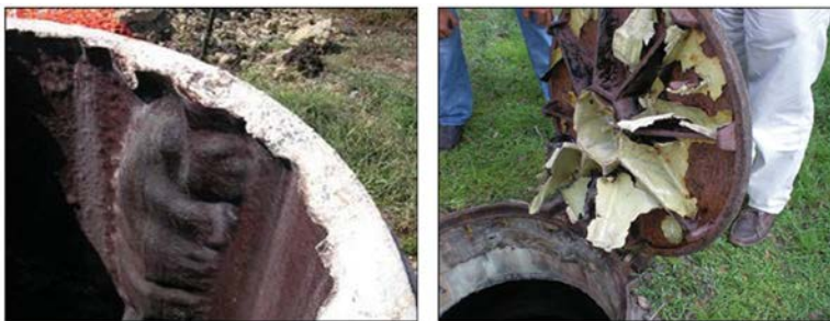
FIG. 14.9. – Observations of a manhole protected with a polymer coating that was not effective in protecting the concrete structure on the left and the steel cover on the right.
