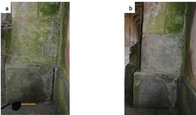
FIG. 15.20. – In situ test, colonized stone pillar: a) before treatment and b) after treatment.
