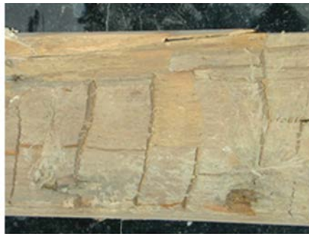
FIG. 15.4. – Appearance of wood panelling damaged by dry rot.
