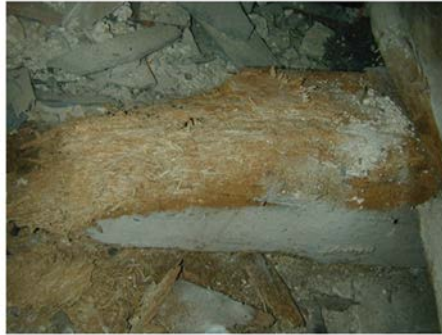
FIG. 15.9. – Damage caused by Phellinus megaloporus .
