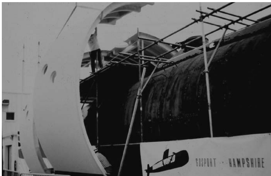
Figure 8 A fibre glass panel being positioned to form a cell around the submarine
