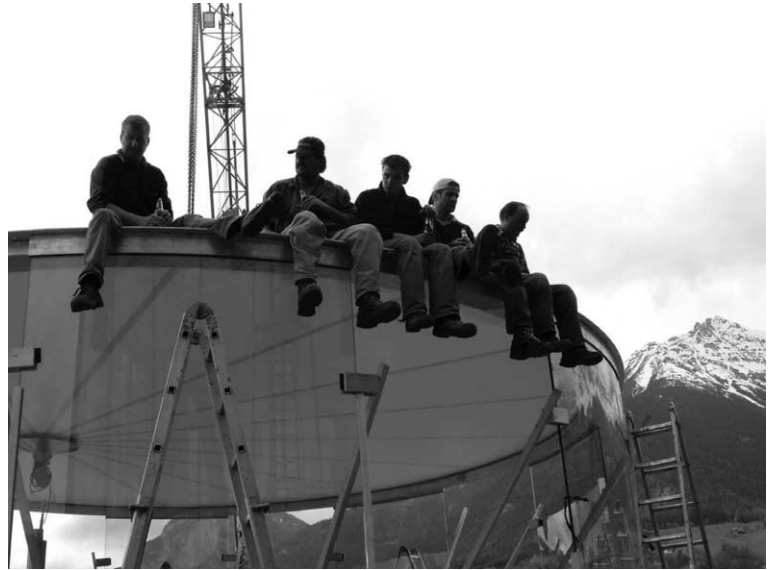
Figure 13 Assembly and test loading of the membrane roof on the free-standing glass panels
