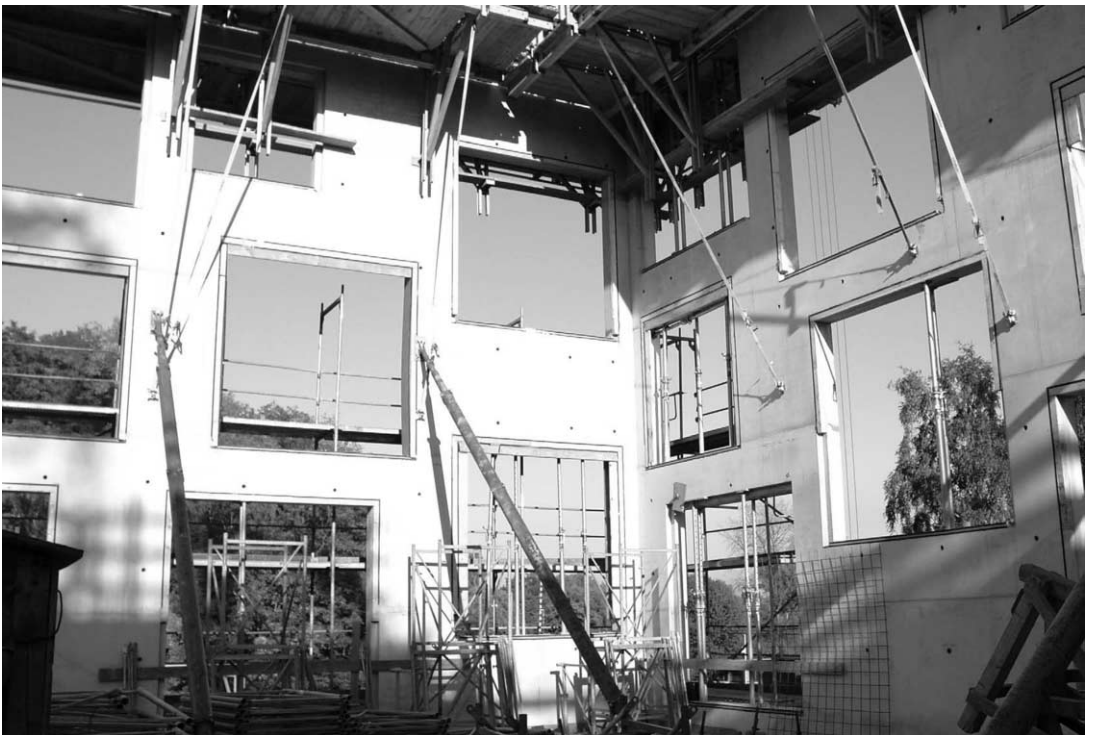
Figure 6 Second floor exterior wall with a free-standing wall during the building process
