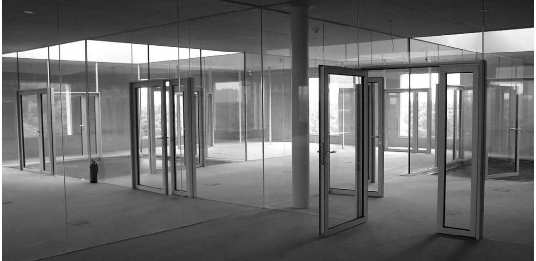
Figure 5 Glass dividing walls with concealed mounting brackets
