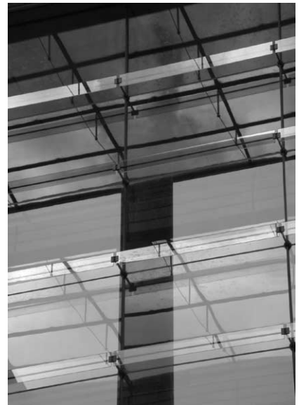
Figure 13-16 Lichthof Facade and Roof German Foreign Ministry, Berlin | Building architect: Müller Reimann Architekten | Engineer: Schlaich, Bergemann & Partner 1999
