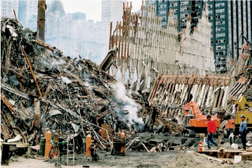
20 FEMA/Bri Rodriguez. Rescue and recovery operations continue at the site of the collapsed World Trade Center, New York (September 26, 2001). Photograph: FEMA.
